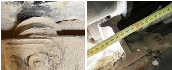
Figure 2. Damaged supporting roller with plateau formation on the running surface (left) and supporting roller flange running against guiding rail (right).
